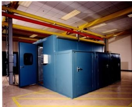
Custom production enclosure containing a M3000-100kj magnetiser
